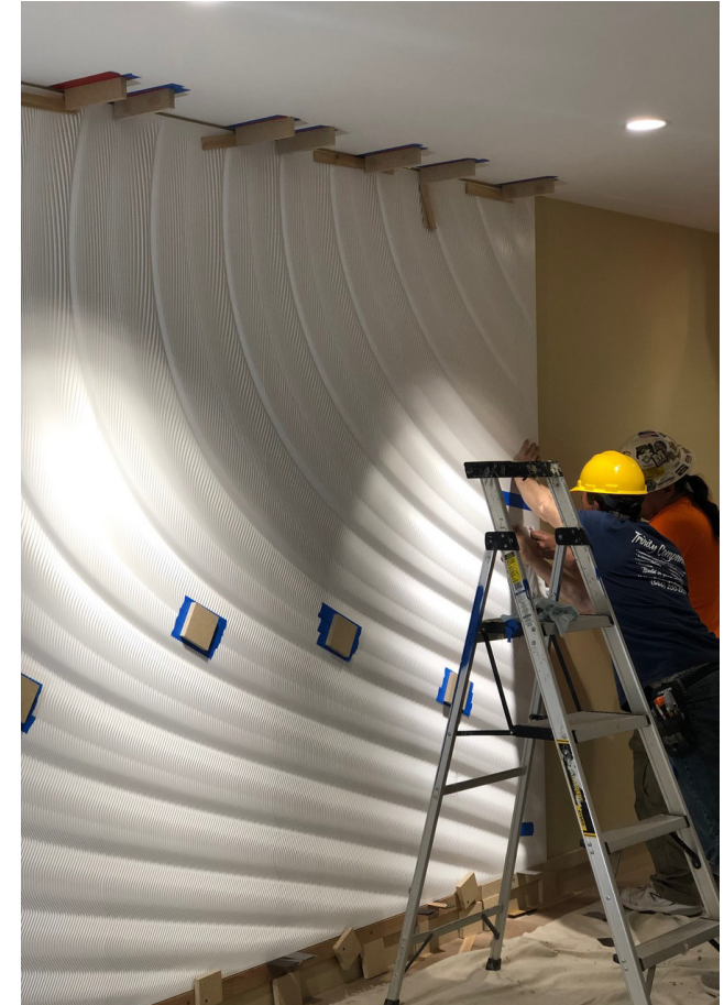
Panels are also held up on top with wood shims to apply pressure above.
