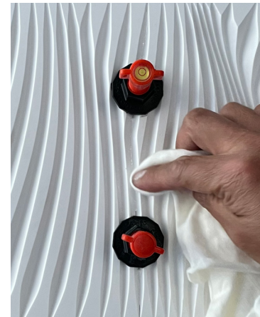
Step 4: With a clean rag, wipe the excess adhesive on the seams.
